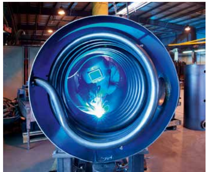
There is a long tradition of metalworking in Brandenburg, like here, at Huch Behälterbau GmbH, which is based in Werder, near Neuruppin. The company has produced items such as tanks for drinking water, heating, and solar equipment since 1928.
